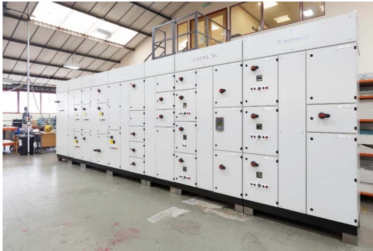
Figure 1 Luano MCC panels at TCL works
