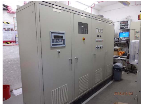
Figure 2 Modified control panel
