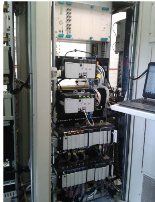
Figure 1 ControlLogix PLC with dual redundant processors
