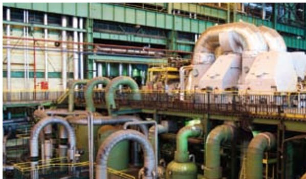
Steam turbine auxiliary plant
