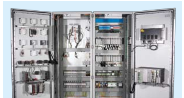
GE Frame 5 control panel
