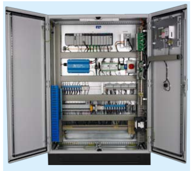
TA control panel
