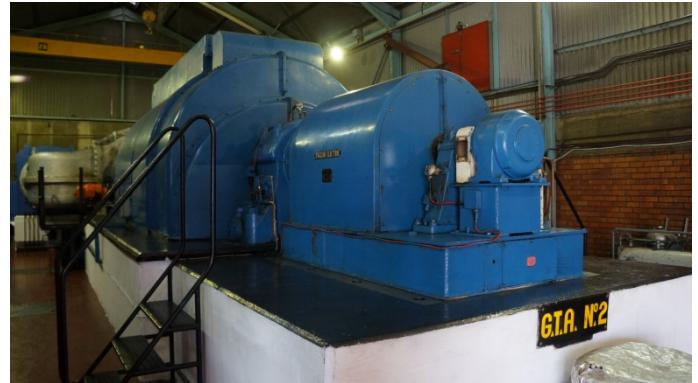
Figure 1 Generator & Exciter before modification
