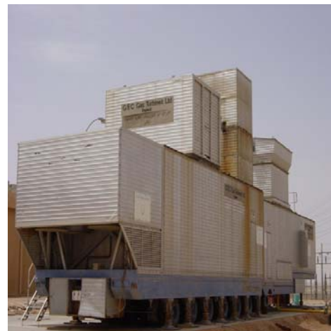
Figure 1 GEC RR Avon mobile generator
